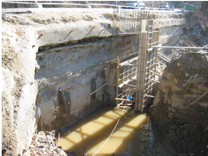
Figure 11 - Finished Soil Nail Wall Showing Weep Holes, the East Abutment of Peirce Mill Dam and the Formwork for the Fishway.
