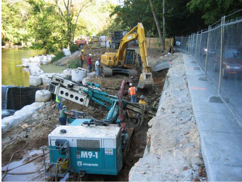
Figure 10 - Soil Nail Installation Showing Proximity of Peirce Mill Dam, Temporary Cofferd Dam and Beach Drive
