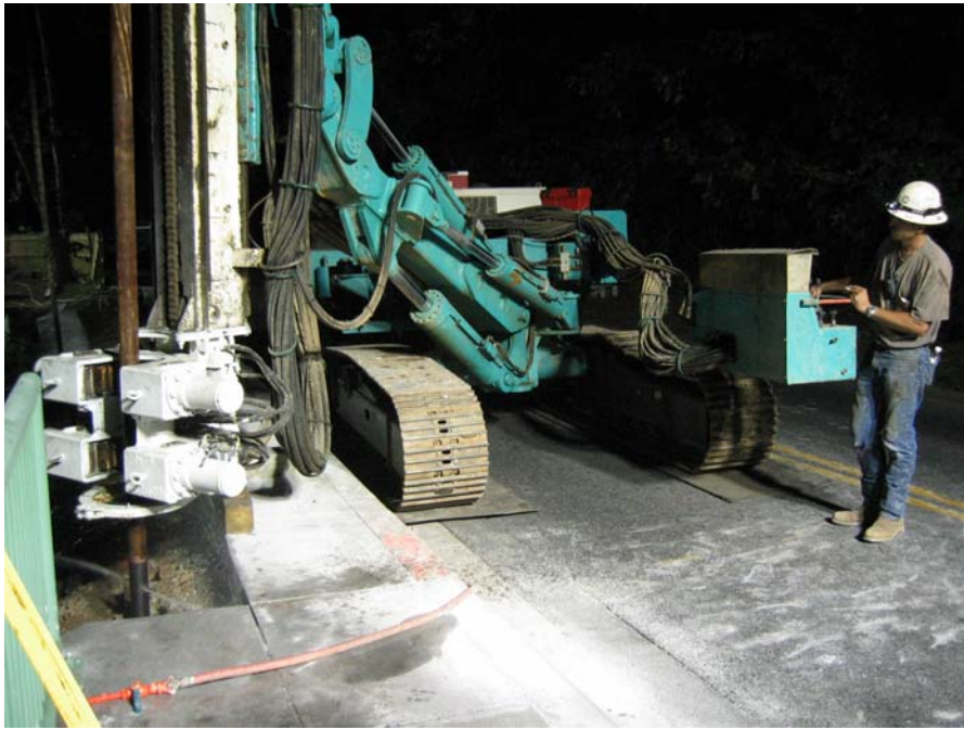
Figure 8 - Jet Grout Installation from Beach Drive Showing Water Jets, Operator and Protective Mats
