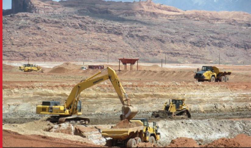
Atlas UMTRA Uranium Mill Tailings Project, Moab, UT. Excavation and transportation by rail of 4 million tons of radioactive mill tailings.
