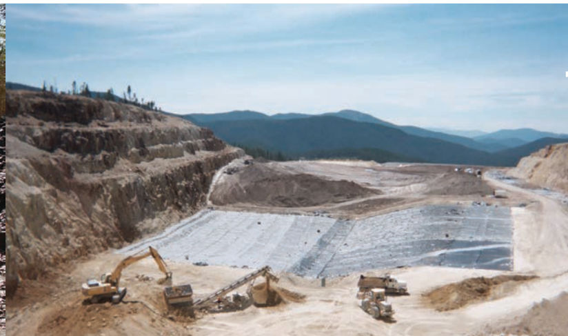
Basin Creek/Luttrell Pit Repository/Upper Ten Mile Creek Acid Mine Reclamation, Rimini, MT. 4-year IDIQ contract for mine reclamation, capping, and wetlands restoration.
