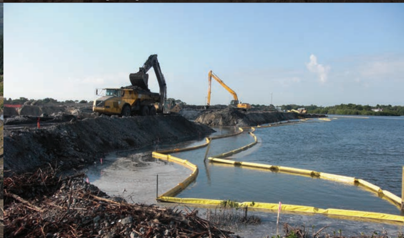
Stauffer Chemical Superfund Site, Tarpon Springs, FL. Excavation of 201,700 cy of pyrophoric phosphate sediments, construction/capping of two RCRA cells, and construction of a 2,800 lf cutoff wall.
