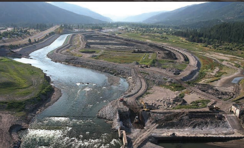
Milltown Dam Superfund Site Remediation, Milltown, MT. Excavation, rail transport, and disposal of 2,200,000 cy of impacted sediments dam and powerhouse demolition, and river restoration.
