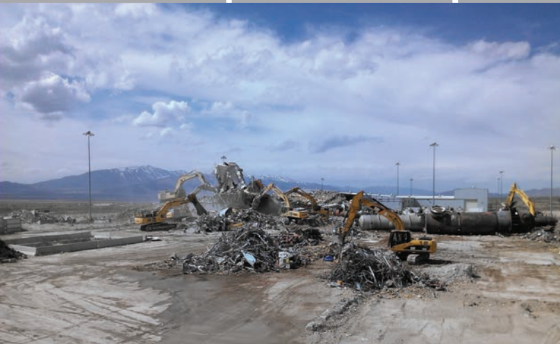
Tooele Chemical Agent Disposal Facility Demolition, Tooele, UT. Demolished over 177,000 sf of structures.
