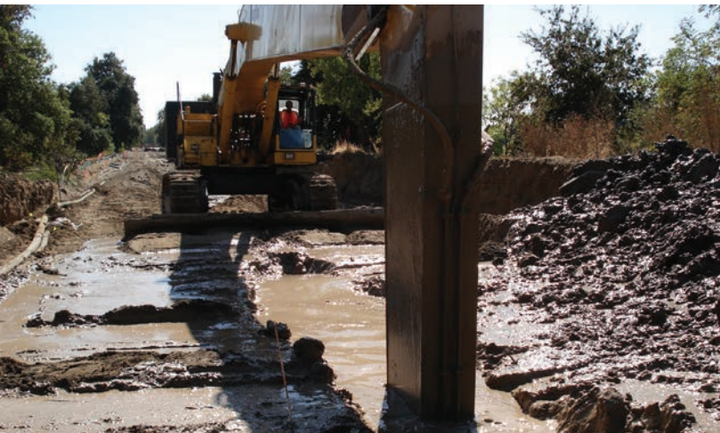
American River Pocket Geotechnical Slurry Wall Project, Sacramento, CA. Construction of two, 100-ft deep slurry walls, USACE South Pacific Division Contractor of the Year.
